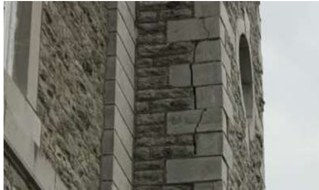
Split in the small bell tower
