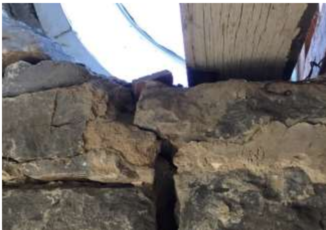
Large crack under tower window
